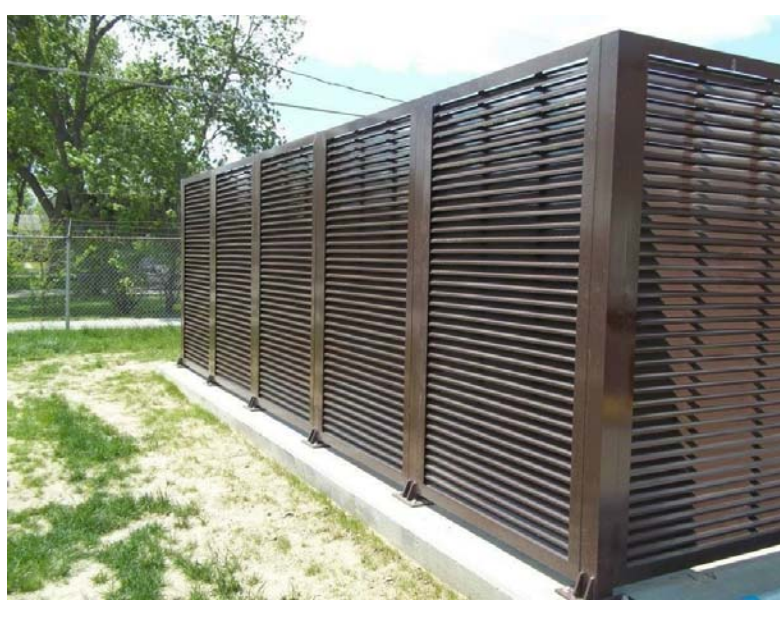
ALUMINUM BLADE SCREENING AT ROOF AND TRANSFORMER
